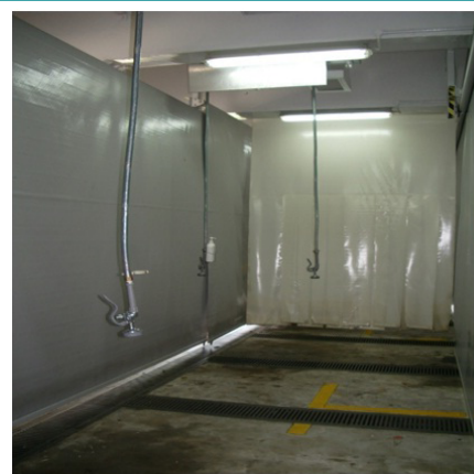
Figure 5. View from the Trolley Shower Lane within the Hospital Decontamination Station (HDS) Showing Water Hose Deployed from the Ceiling upon Activation
