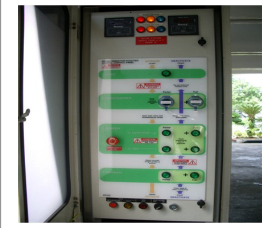
Figure 4. Control panel for activation of Hospital Decontamination Station with Options for Partial or Full Deployment
